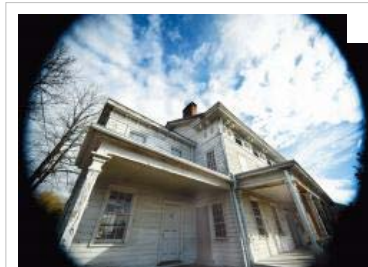
Top: Denny Caruso looks over the work being done in Lakeview's basement, where workers had to stabilize the walls to prevent them from caving in.
