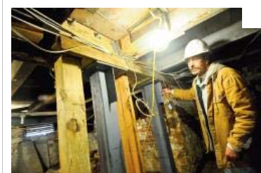
Above: Denny Caruso points out the steel structural supports installed in the basement. Below: Shutters are tagged to show where each was located on the outside of the mansion. Aesthetic improvements will take place once the building is made
