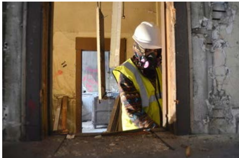
Jesus Lopez of WU & Associates removes debris from the Glassboro train station, which restoration began to return the station to its original state, Tuesday, Feb. 5, 2013. (Staff Photo by Tom Scott/South Jersey Times)
